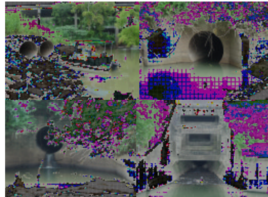
Figure 25. UL. Shepherd stormwater outfall. UR. North Waugh stormwater outfall. LL. South Waugh stormwater outfall. LR. Sabine stormwater outfall.
