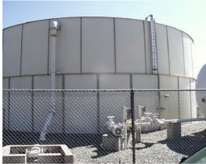
Los Molinos Community Services District Small Water System Well and Storage
