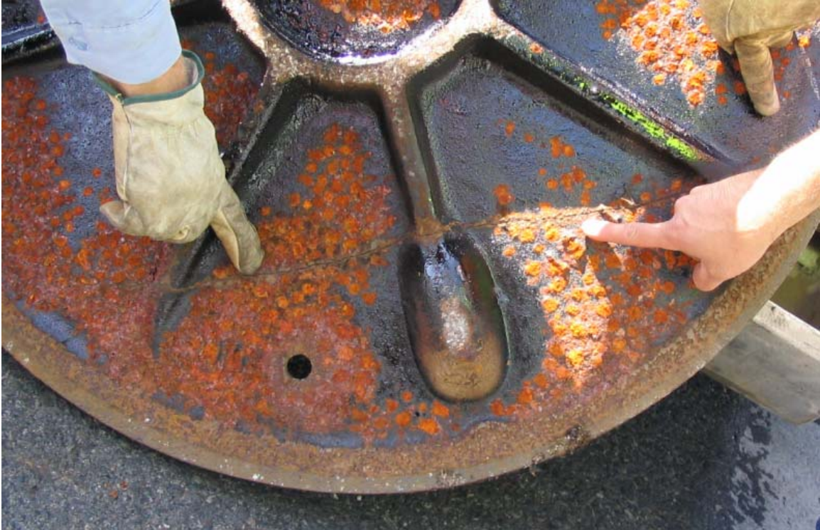
Figure 22 – Cracked cover replaced by crew
