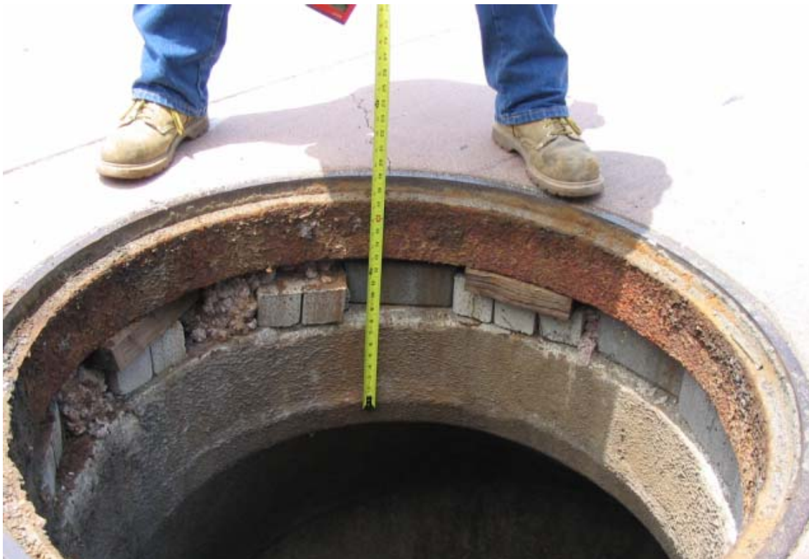
Figure 11 – Wood used to support frame; settling and surface cracks are visible
