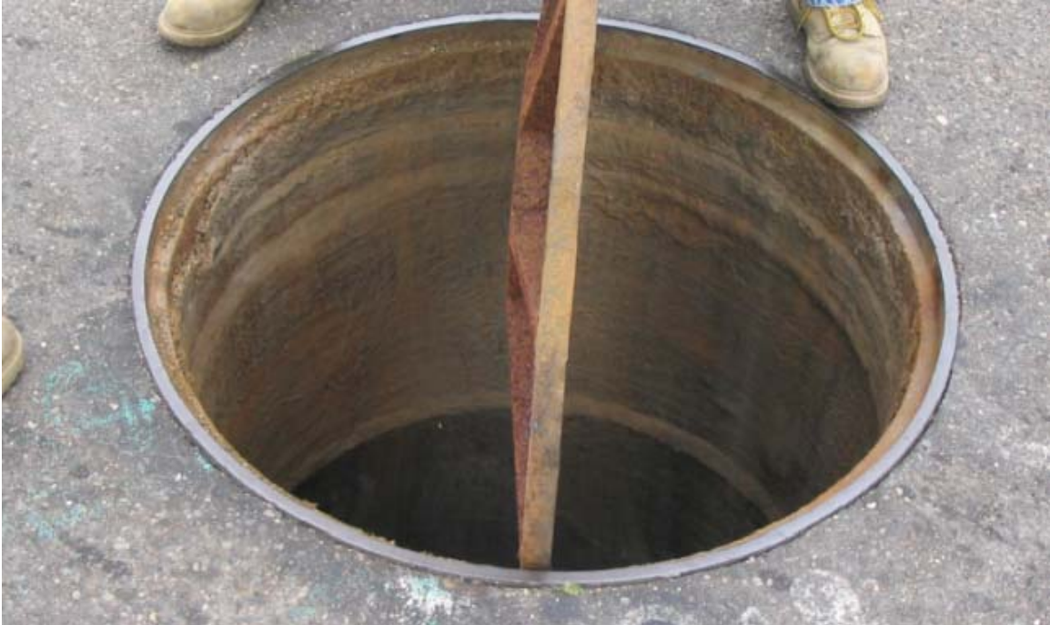
Figure 15 - Polyurethane coated manhole structure in Dyer Rd.
