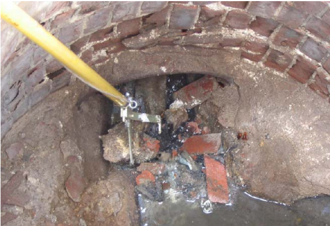
Figure 19 – Debris restricting flow
