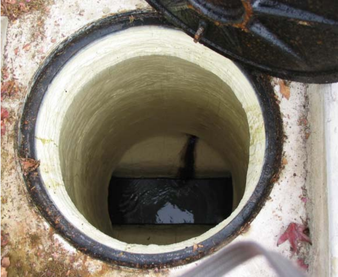
Figure 14 – Polyurethane coated manhole structure
