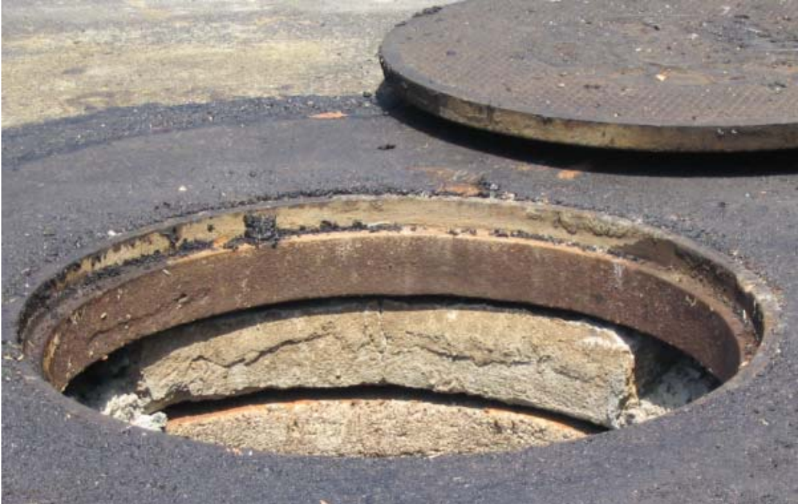
Figure 12 – broken grade ring and joints not filled with mortar
