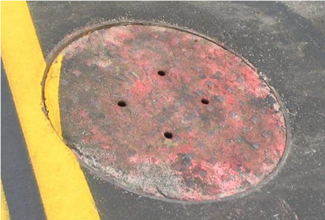
Figure 6 – Worn City of Fullerton frame and cover
