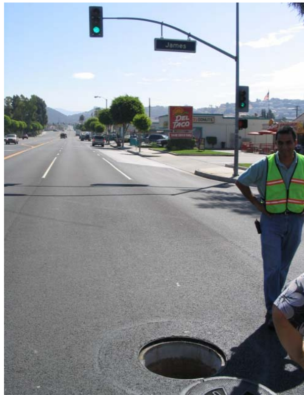
Figure 10 – Structure raised at Chapman and James after the contractor was notified
