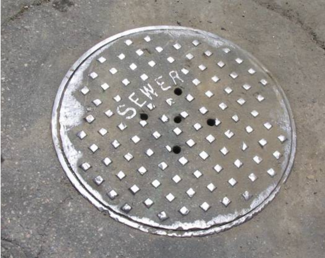
Figure 1 – Worn OCSD frame and cover
