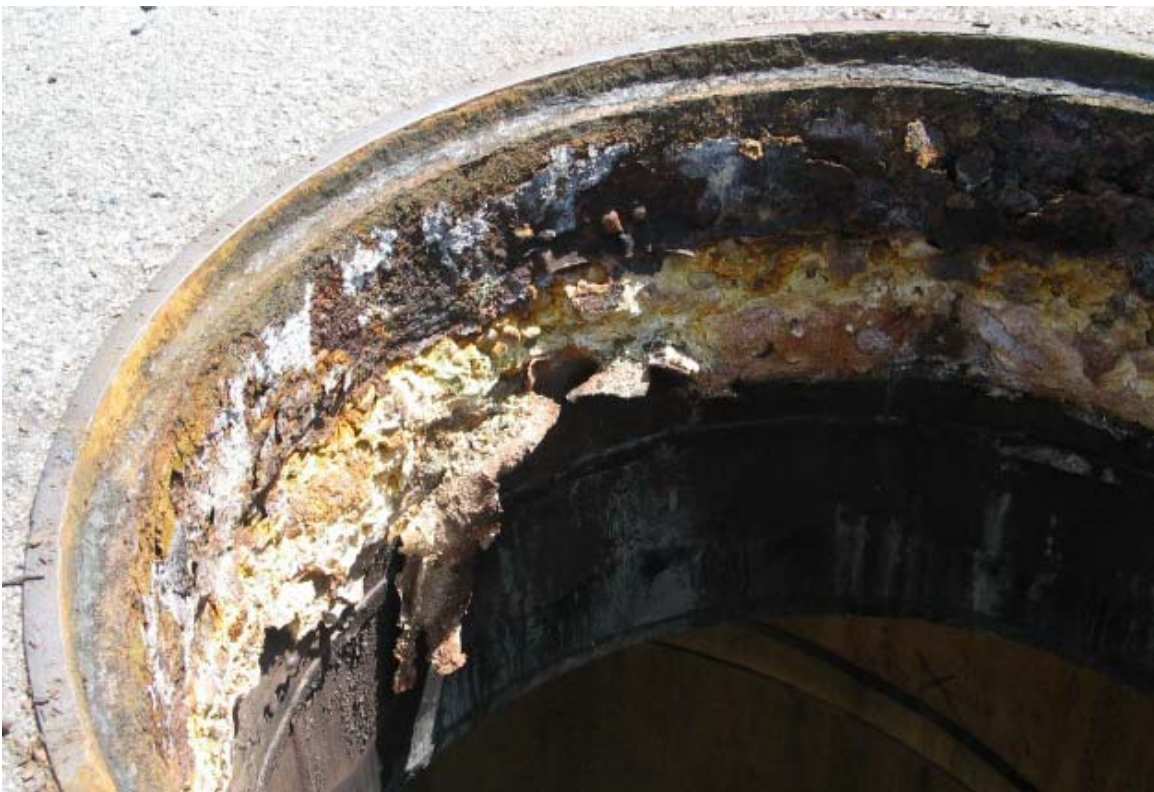
Figure 21 – Failed PVC coating as the result of prior street-overlay
