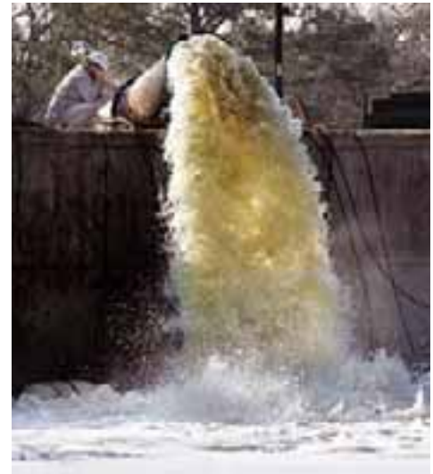
Figure 2: Portable Pump Operation
