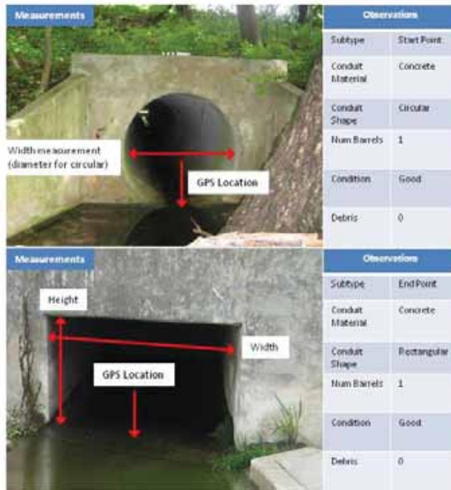
Figure 6 Culvert Collection Examples
