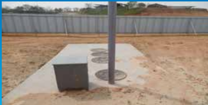
waste water processing facilities
