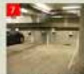
Electric Vehicle Charging Station
