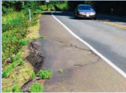
Embankment pop outs
